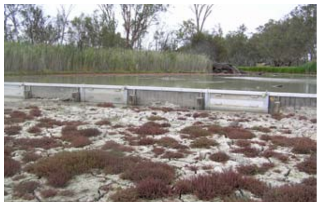
ABOVE (TOP) Construction was carried out almost entirely from the barge using an excavator fitted with a pile driver. A steel frame was constructed initially to guide the construction.
