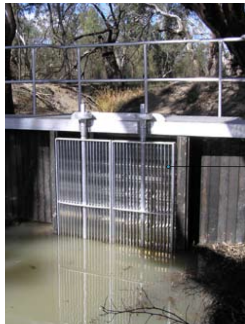
Rotary carp screens prevent large carp from entering the lagoon.
